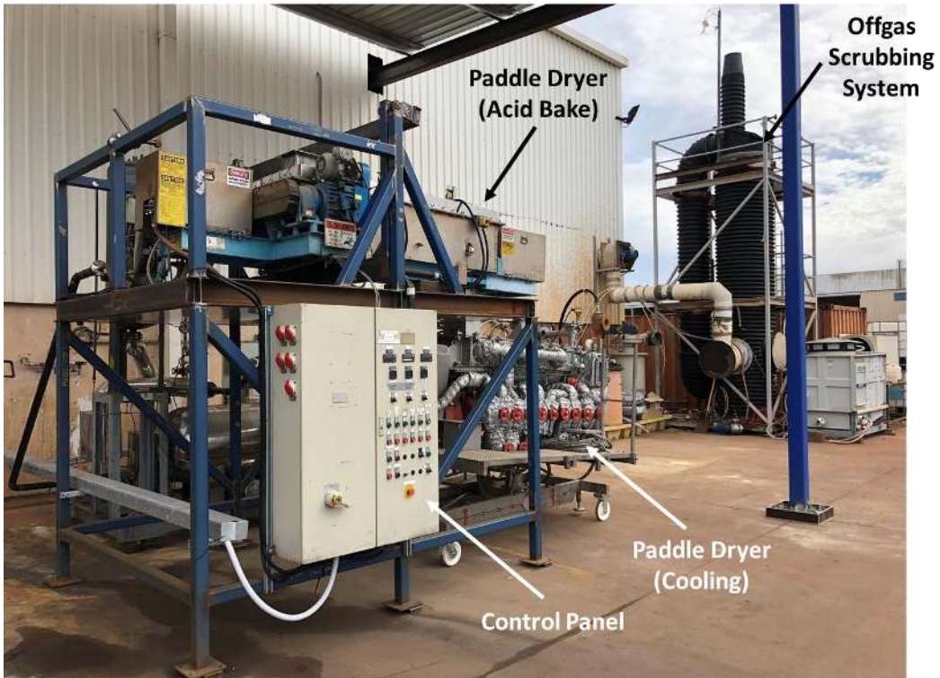
Figure 1b: Phase 4 Acid Bake Pilot Plant at SGS Awaiting Installation of PLR Feeder and Pug Mixer
