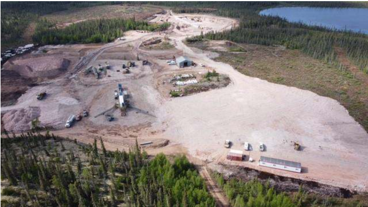
Overhead image of site with ore sorter in the foreground and pit in the background
