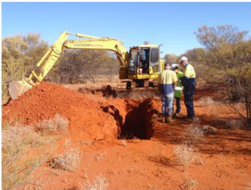
Figure 2: Geotechnical test pit excavation at the site of the Nolans process plant
