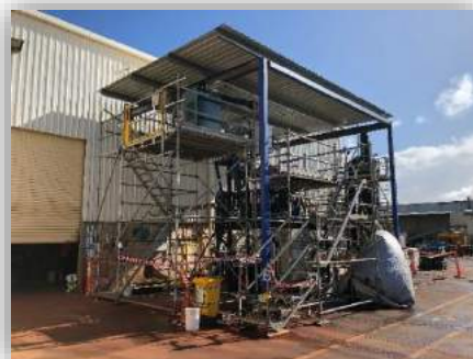
Acid Bake Pilot Plant
