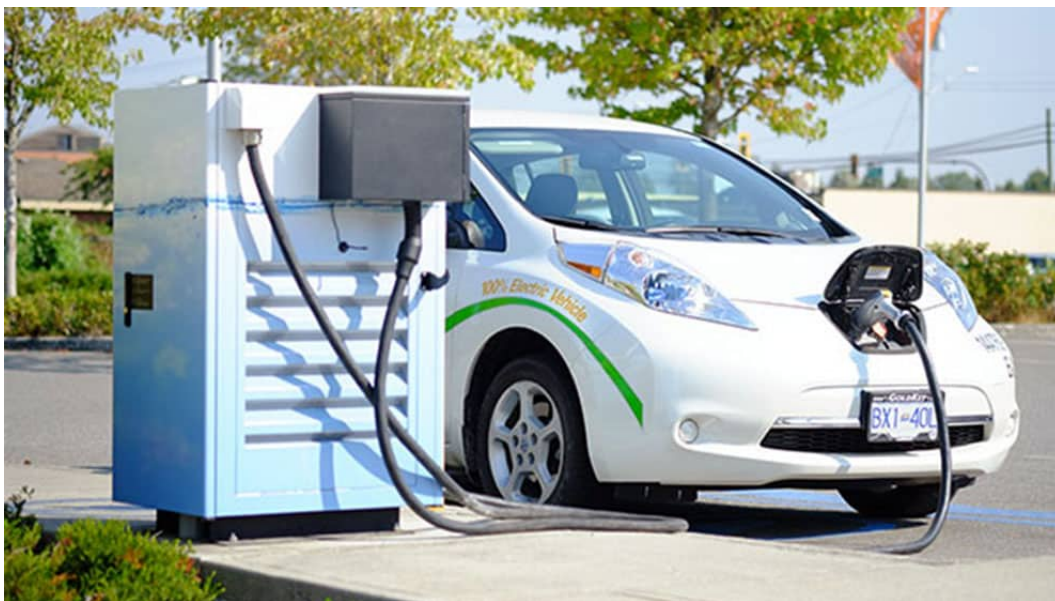
Recharging an EV
